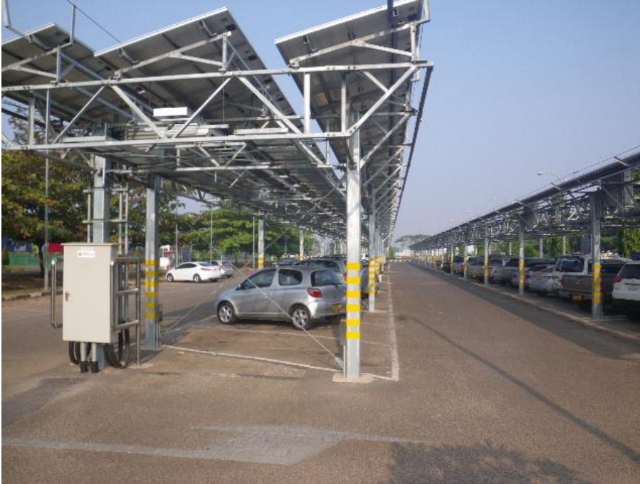
the PV System in the Vientiane international Airport 236 kWh
