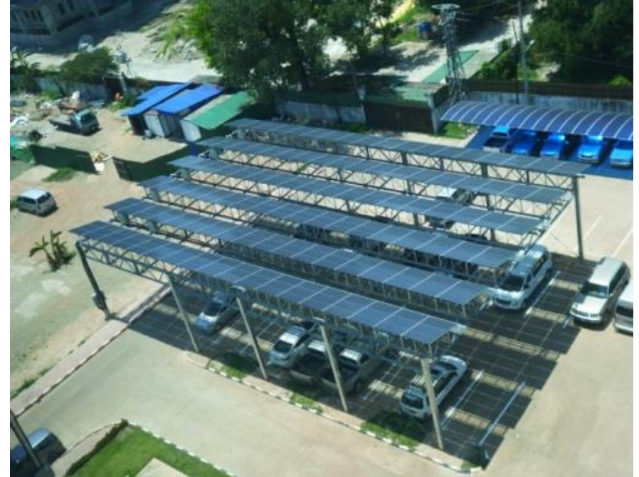
the PV System in EDL Headquarter 178 kWh
